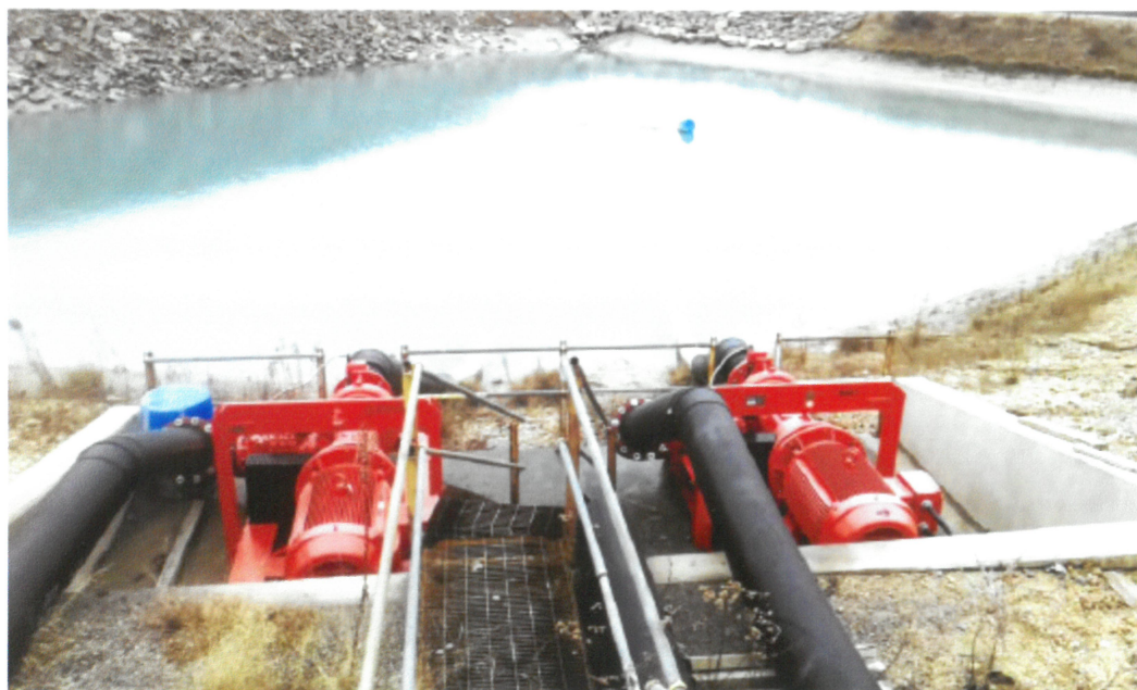
Each of these twin Godwin 12-inch pumps delivers 4300 gallons per minute of water. Middleport has five ponds totaling more than 10 million gallons of water reserve for quarry needs.
